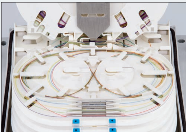
Fiber handling in SC cassette
